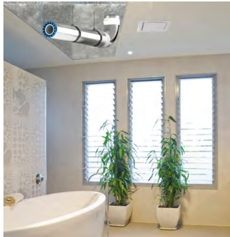
Lagged PVC Pipe (Soundlag)
