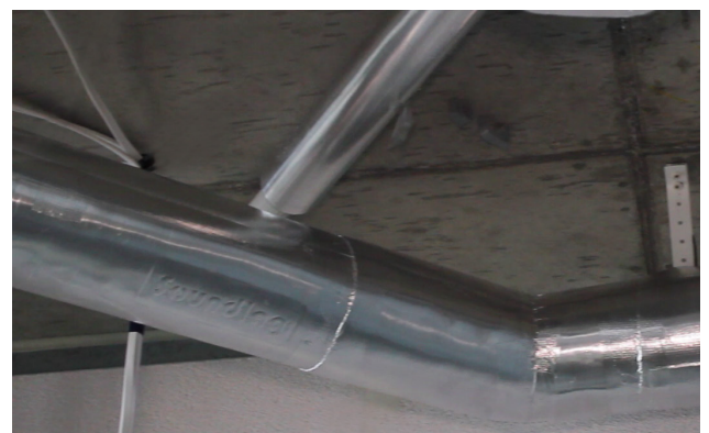
View of Soundlag installed above ceiling below residential apartments
