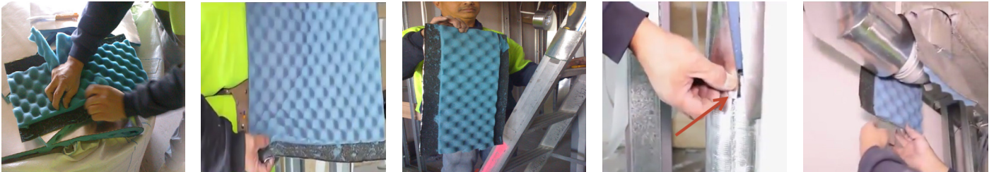
Images (left to right) show the removal of foam before being overlapped at joints. Joints overlapped without foam removal provide a smooth surface.
